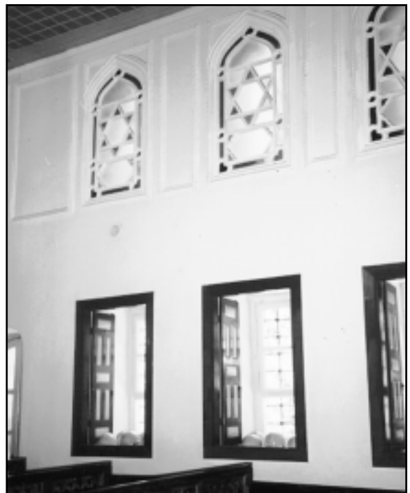
Interior, Achrida Synagogue, Istanbul (Notice hardhats on window sills, used in case of earthquakes)
